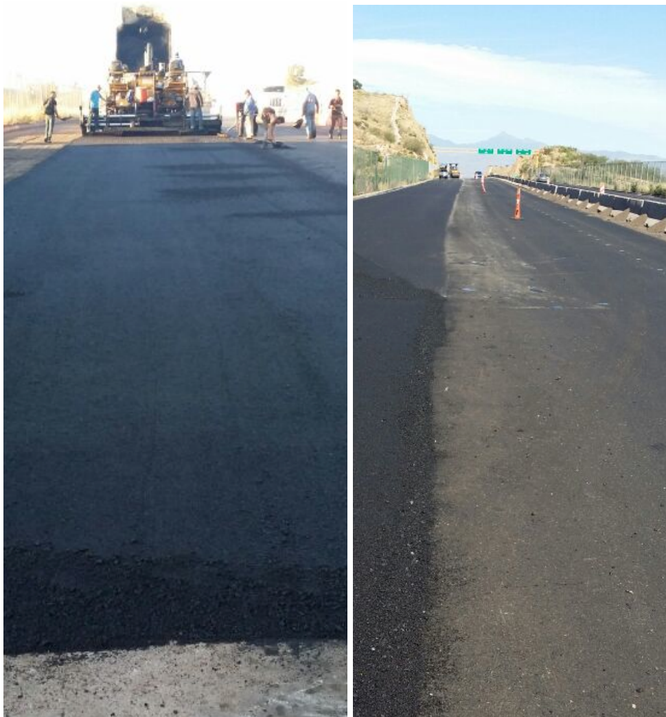
Photos of the progress being made for the repaving of the Corridor, including the signage that has been installed.
